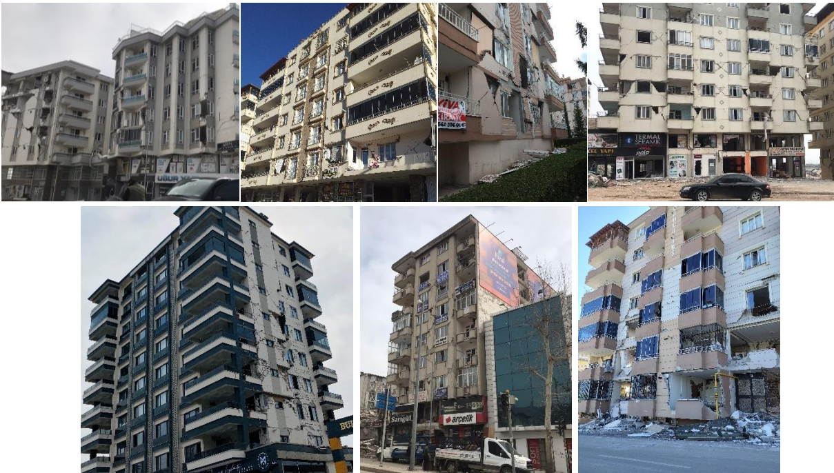
Figure 1.1. Various examples of infill wall damage
