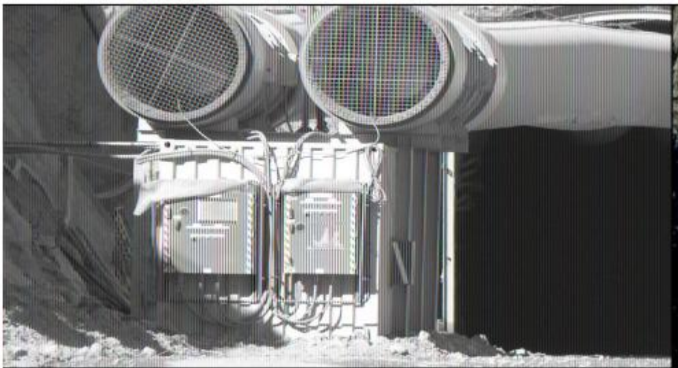
Figure.3. Suction type fan for ventilation and discharging harmful gases Aydın, G., & Karakurt, İ. (2021)
